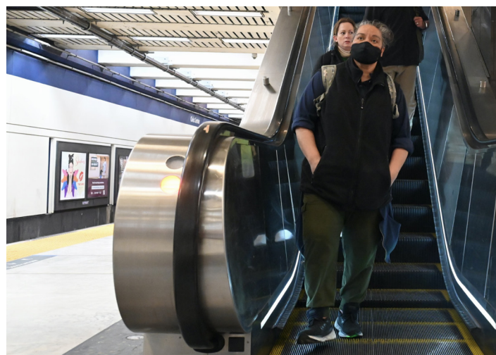
BART's new escalators are more energy efficient, with LED lighting, a "sleep mode," and variable frequency regenerative drives.
