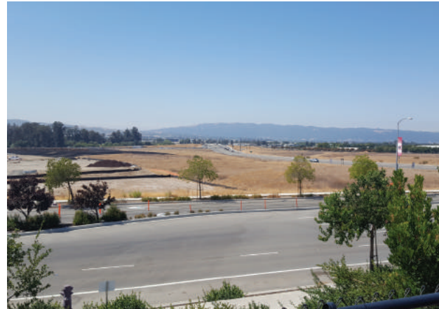
Looking south from Portola Avenue, view of Isabel North Area (center) with Shea Homes-Sage Project under construction (left).
